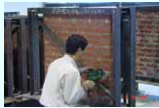
2. Drilling holes through the masonry wall in case of existing structure but in case of new construction we can put straws to make holes
